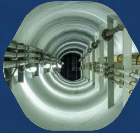
Underground Electric System
